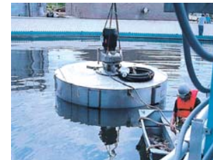
Oxygen for wastewater treatment
