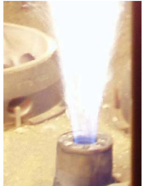
'A' burner fired in heater.
